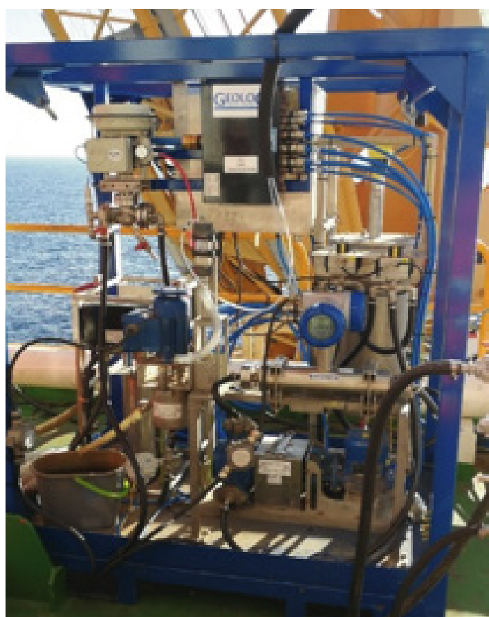
Fig.2: Pressure control, regulator and gas extractor
